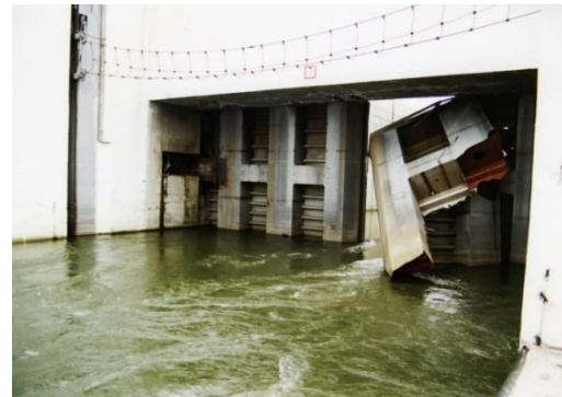
Example of the Damage to the Lower Gate (Inappropriate Material Wear) from the Late 90s.
