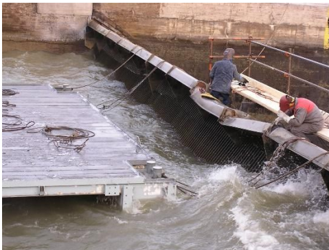
Example of the Damage to the Upper Gate Caused by a Ship Collision.
